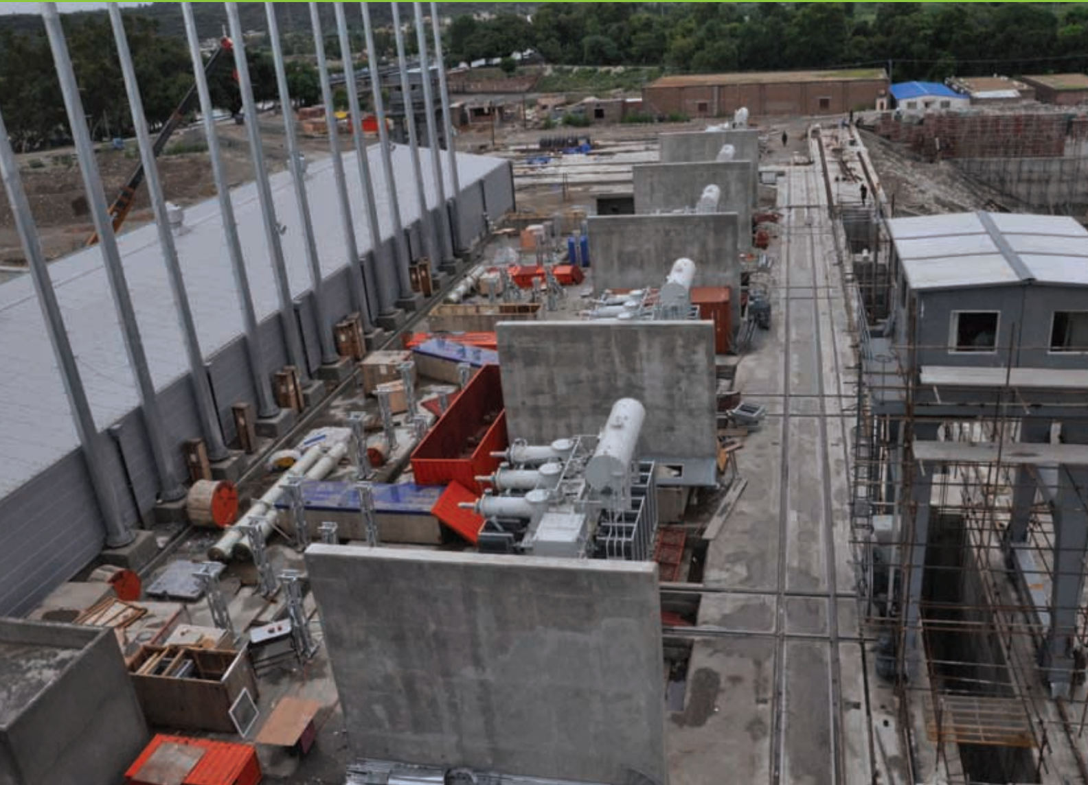
View of Laraib Plant
